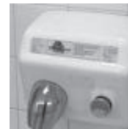
Hand drier in toilet
